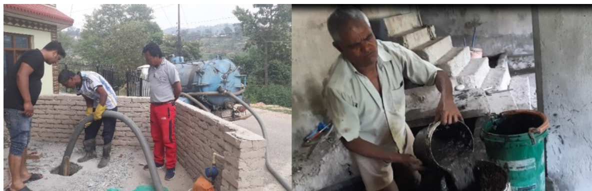
Figure 8: Containment being emptied mechanically and manually in Dhulikhel municipality.
