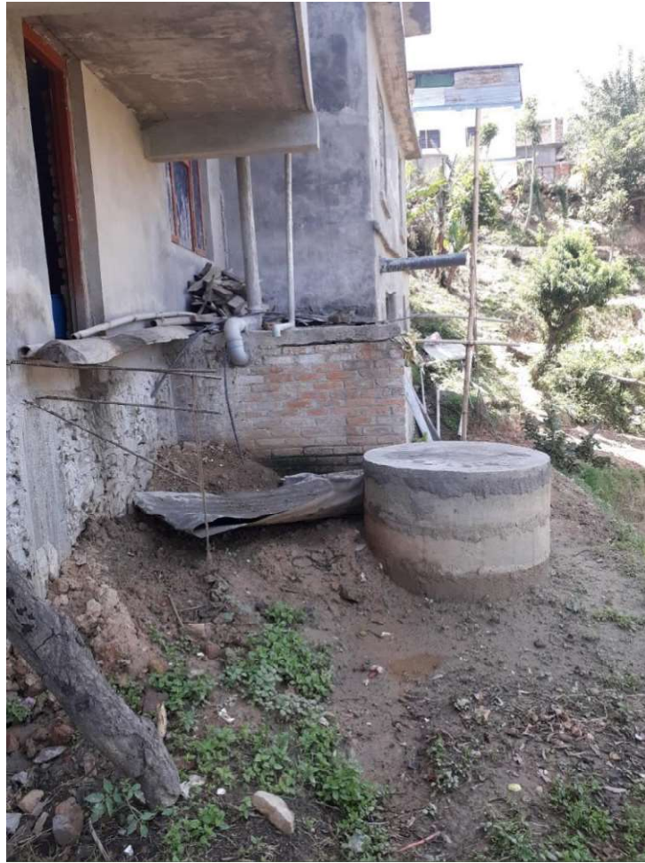
Figure 7: A concrete single pit installed at households in Dhulikhel municipality.
