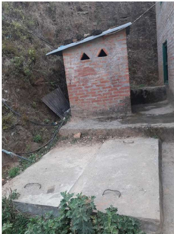
Figure 6: Fully lined tank at household in Dhulikhel municipality.
