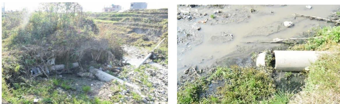
Figure 2: Damaged and disconnected river crossings for sewer networks.
