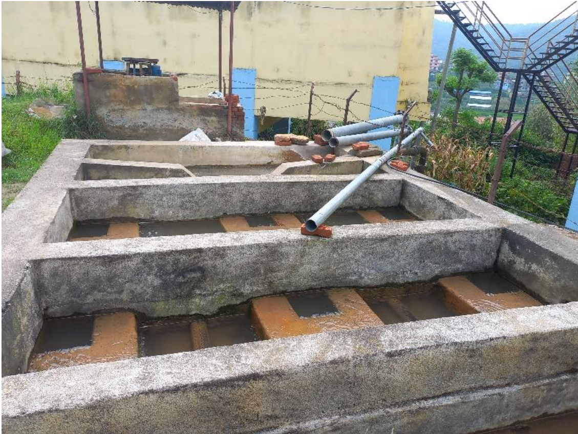
Figure 13: Sedimentation unit in water supply schemes operated by NWSC.
