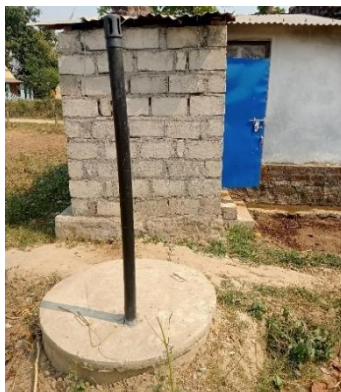
Figure 9: Toilet connected to lined pit with semi-permeable walls and open bottom at a household.
