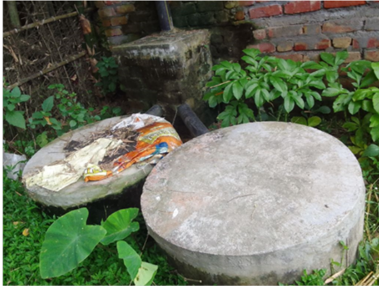
Figure 4: Inappropriate design of the twin pits, where the distance between two pits is less than 1.2 m.
