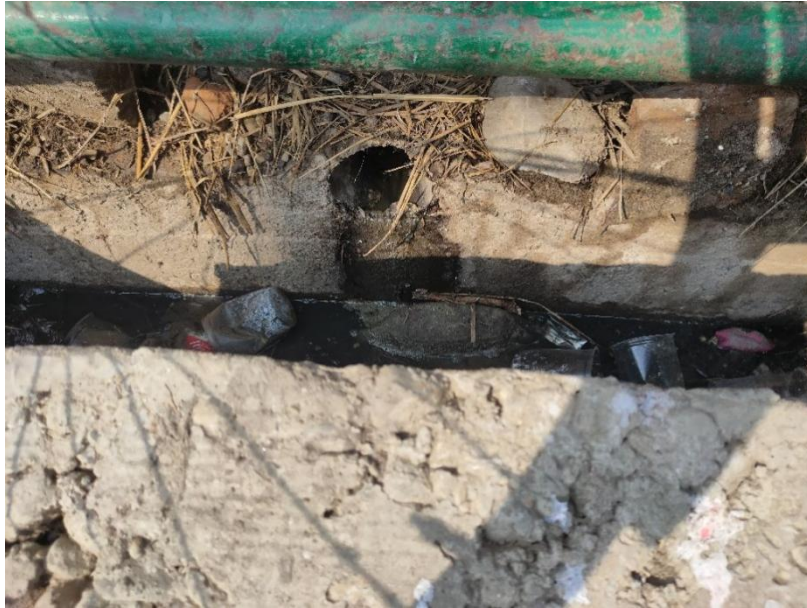
Figure 6: A discharge of effluent from containment to an open drain.
