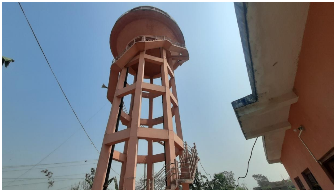
Figure 14: Overhead tank of Siswa WSUC.
