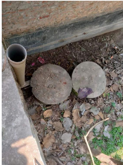
Figure 4: Inappropriate design of the twin pits, where the distance between two pits is less than 1.2 m
