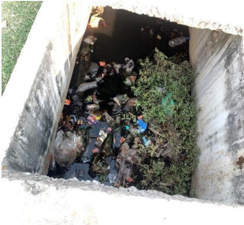
Figure 3: Wastewater being disposed of directly in stormwater drainage.
