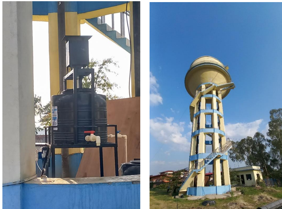
Figure 18: Overhead water tank along with automatic chlorination unit.
