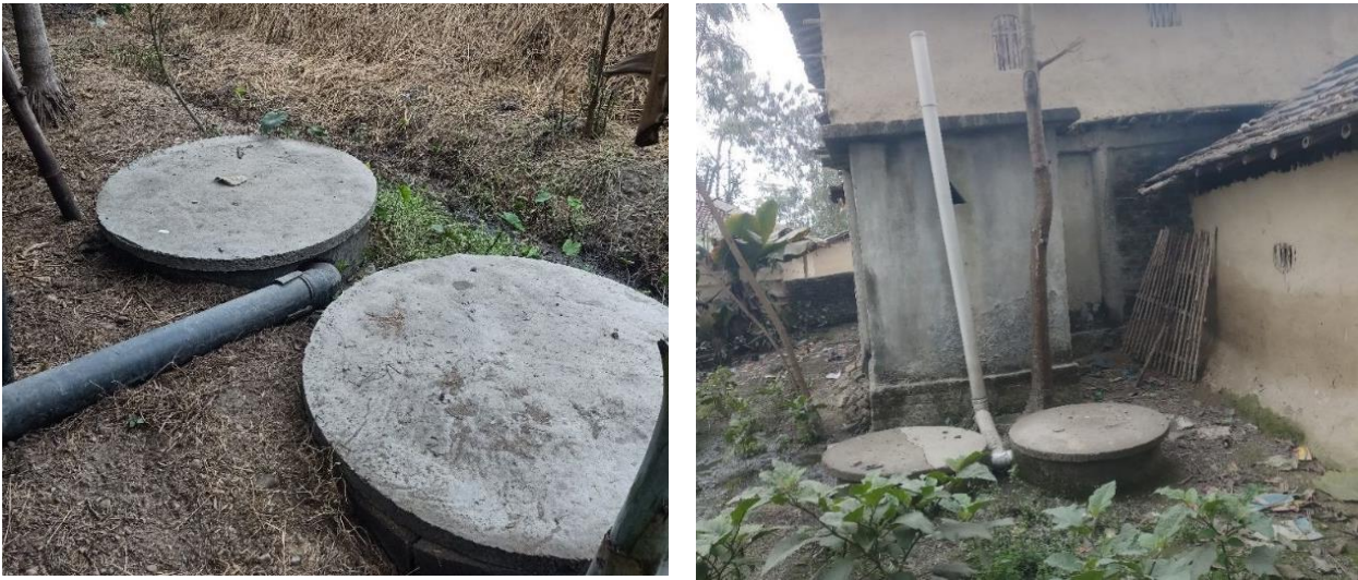
Figure 8: Inappropriate design of twin pits, the distance between two pits is less than 1.2m
