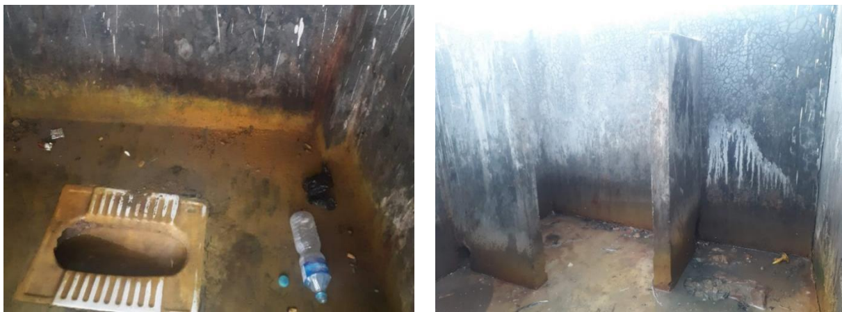
Figure 12: Status of pan (left) and urinals in female compartment (right) of public toilet at local marketplace of ward no.2.
