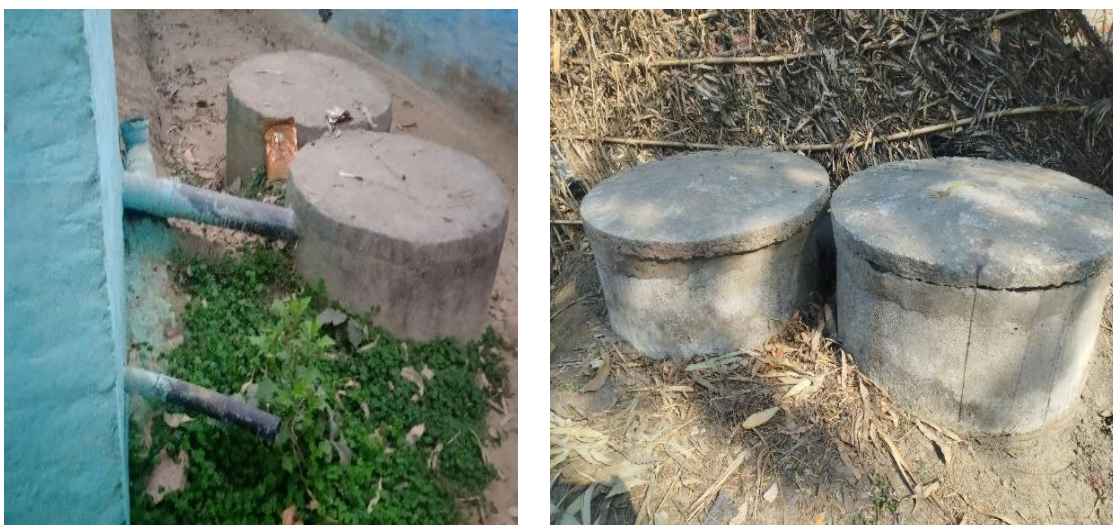
Figure 2: Inappropriate design of the twin pits.
