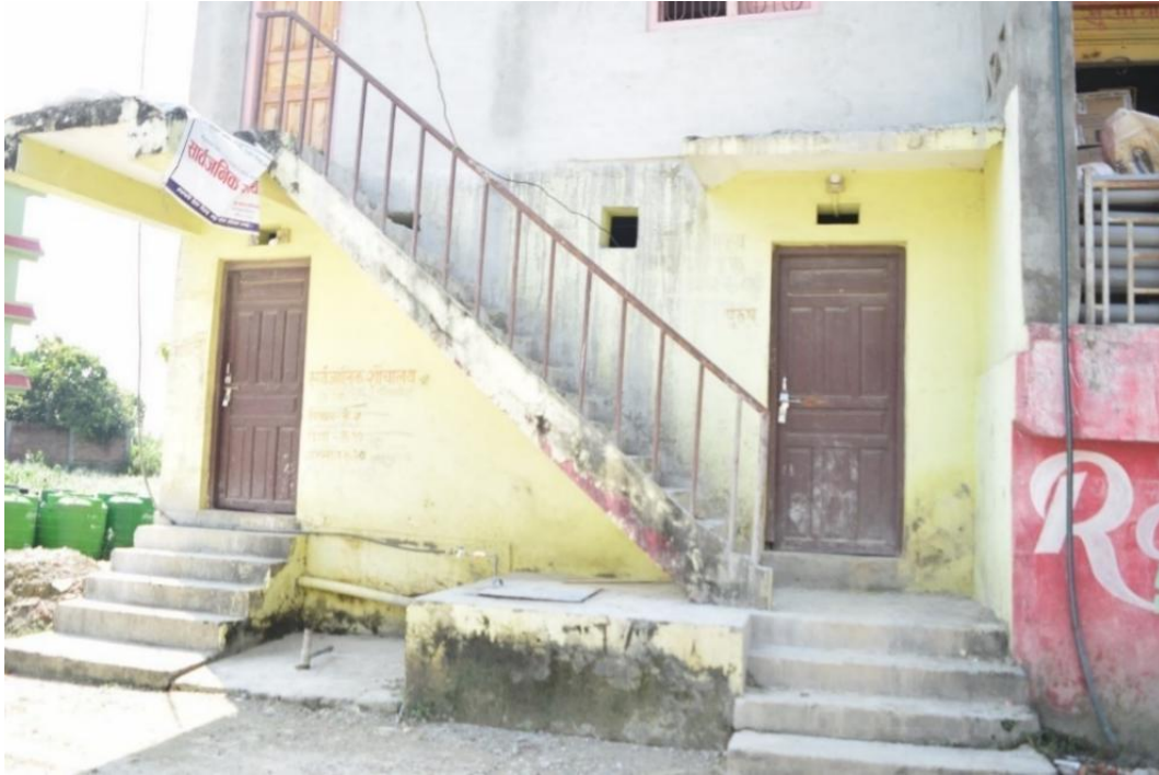
Figure 12: Non-functional public toilet at Katari chowk.
