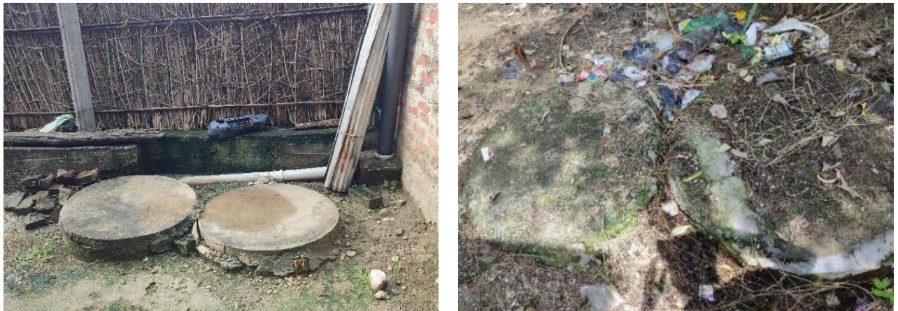
Figure 7: Inappropriate design of twin pits, the distance between two pits is less than 1.2m.
