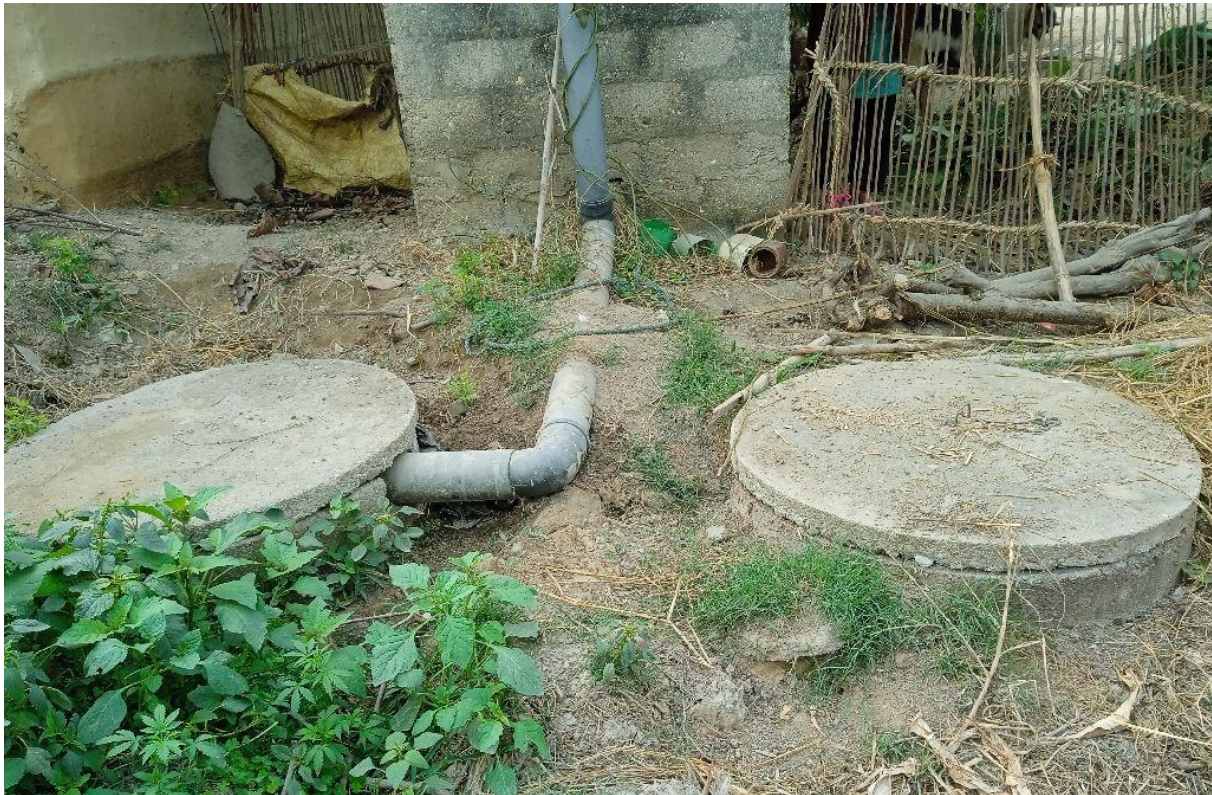
Figure 6: Inappropriate design of the twin pits, where the distance between two pits is less than 1 m.
