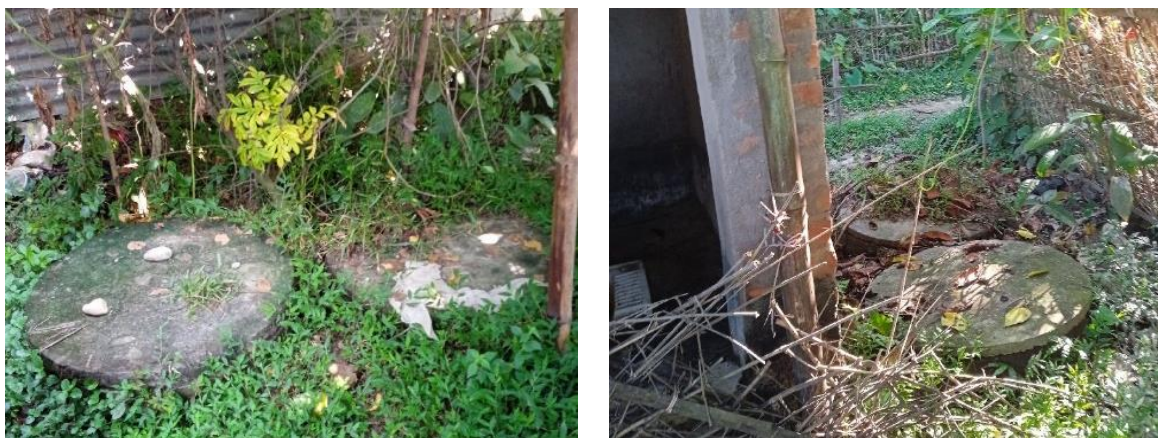
Figure 5: Inappropriate design of twin pits, the distance between two pits is less than 1.2m.
