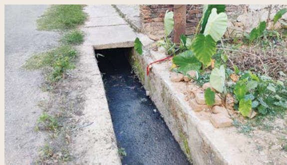
Toilet directly connected to an open drain.
