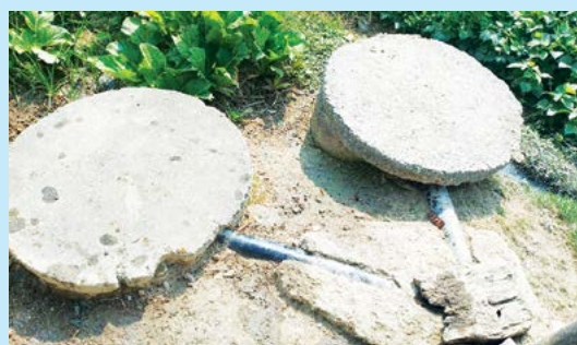
Twin pit installed in sampled HH
