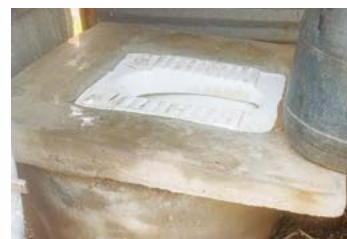
Direct pit installed in one of the sampled HH
