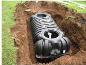
Readymade plastic septic tank
