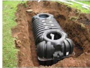
Readymade plastic septic tank
